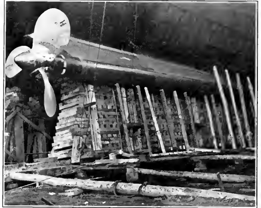
After poppet built up with 7 \frac{1}{2} x 12 pine planks with two longitudinal layers to each transverse layer. The propeller is designed to transmit 13,250 horsepower at 125 revolutions per minute.
